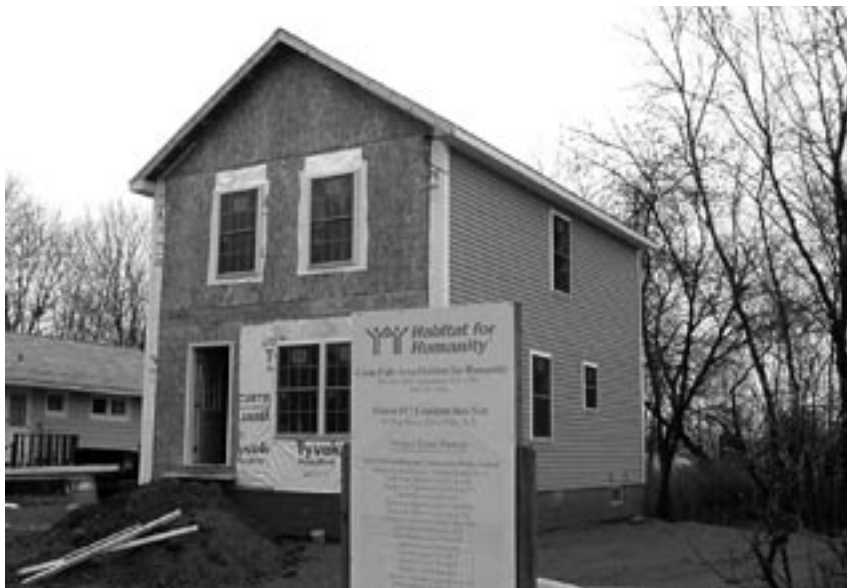
79 Platt Street – Framing and siding are completed along with utility services. Interior utility rough-in work can now begin.
